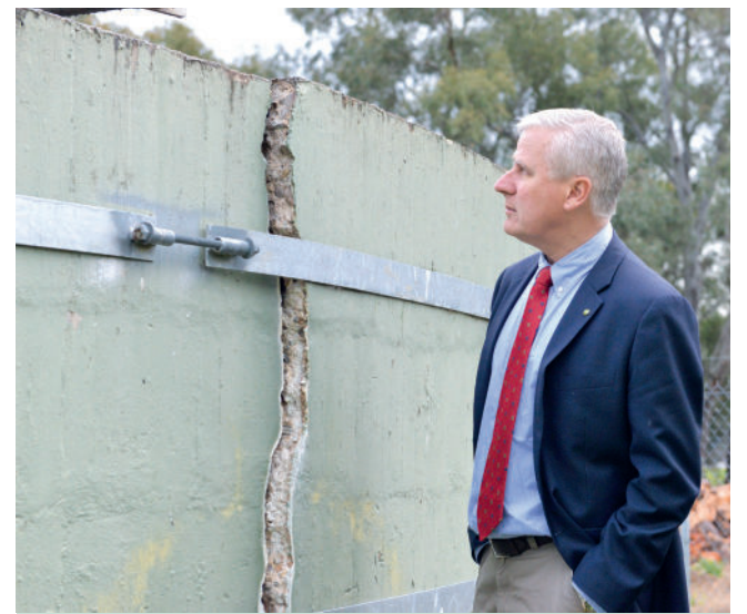
BADLY NEEDED: Inspecting the state of the current infrastructure at Gundagai's sewage treatment plant. Funding of $3.5 million has been secured for Cootamundra-Gundagai Regional Council towards building a new plant.
